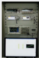
CEDM Coil Current Constant Monitoring System
