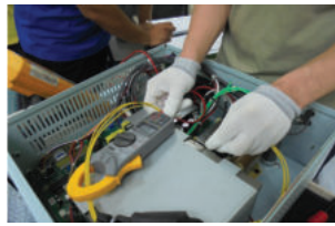
UPS integrity test
